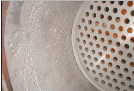
After cleaning and decontamination, ARC 858 is applied to fill and smooth surface
