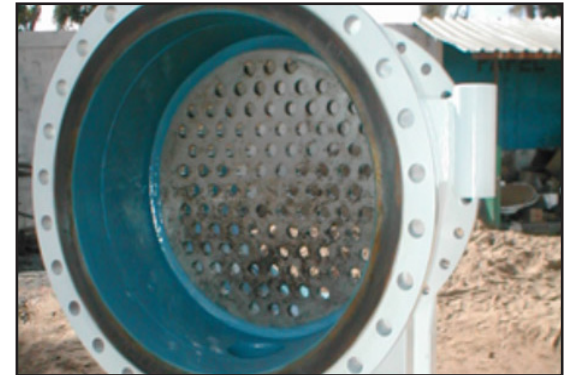
After cleaning and decontamination, ARC 858 is applied to fill and smooth surface
