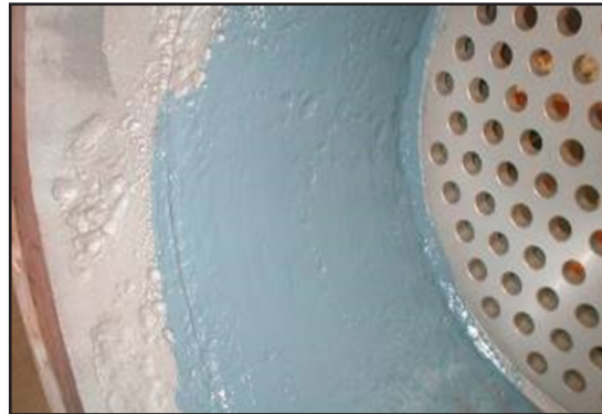
After application of ARC 858, ARC SD4i is applied for protection and enhanced flow efficiency
